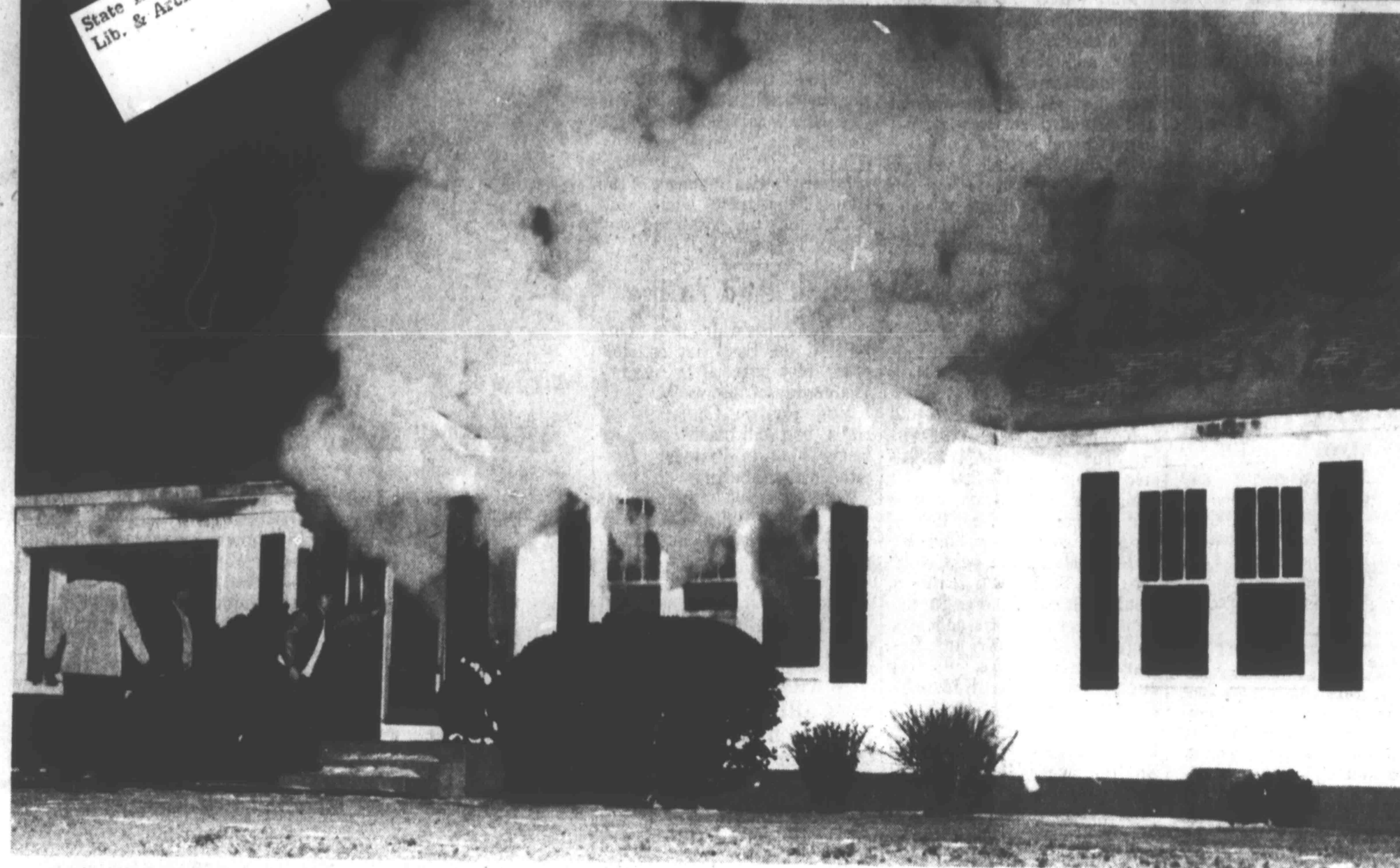
THE HOME OF MAGISTRATE LAWSON ELDER on Cedar Grove Road near Ripley suffered severe interior damage from fire which broke out about 8 p.m. Sunday—it is believed from a furnace—in zero degree weather which hampered fire-fighters from Halls and Ripley. No one was home when the blaze started. The Jimmy Hensley home in Cedar Grove Sub-Division near Ripley was destroyed last Friday after a log rolled from a fire-place, and Oscar Griggs' home in Morris Sub-Division near Arp suffered minor damage about 8 a.m. Tuesday when a blaze resulted from attempts to thaw out frozen water pipes, Ripley firemen reported.
